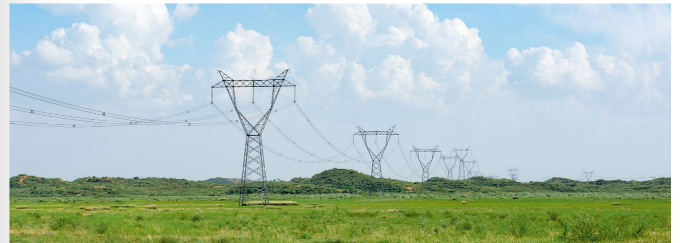
Figure 2: UHV power transmission
