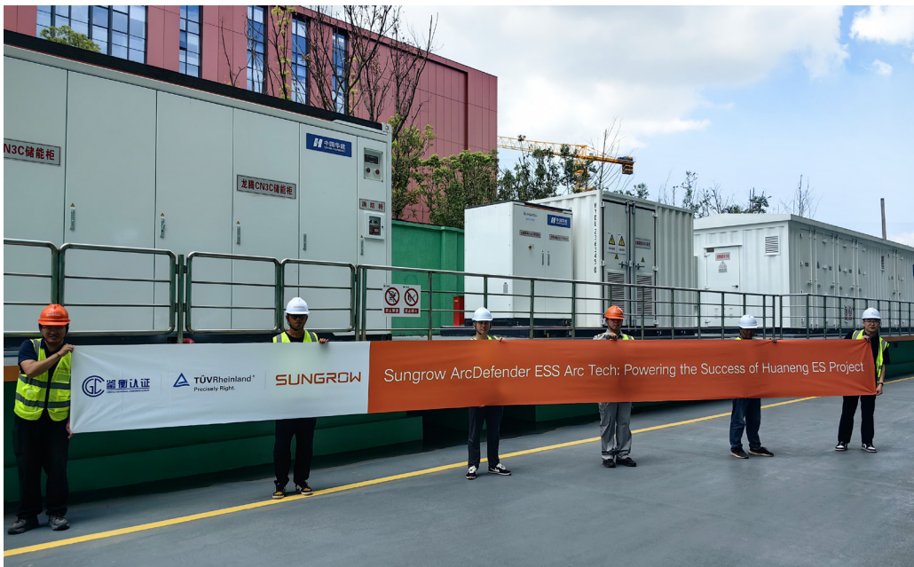
Figure 24 ArcDefender™ technology successfully applied in Huaneng Longteng ESS project
